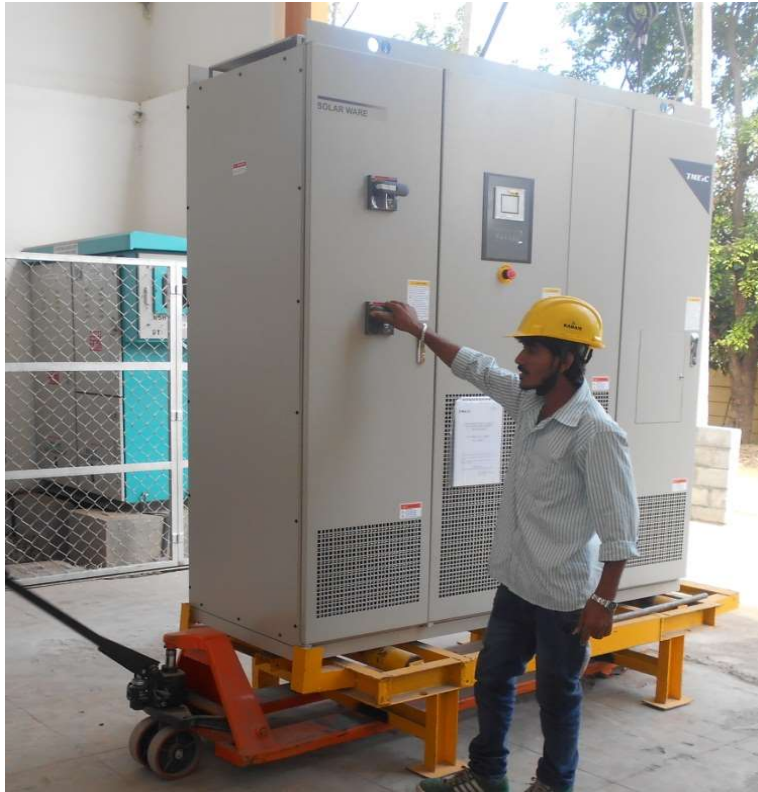
Panel handling facility
