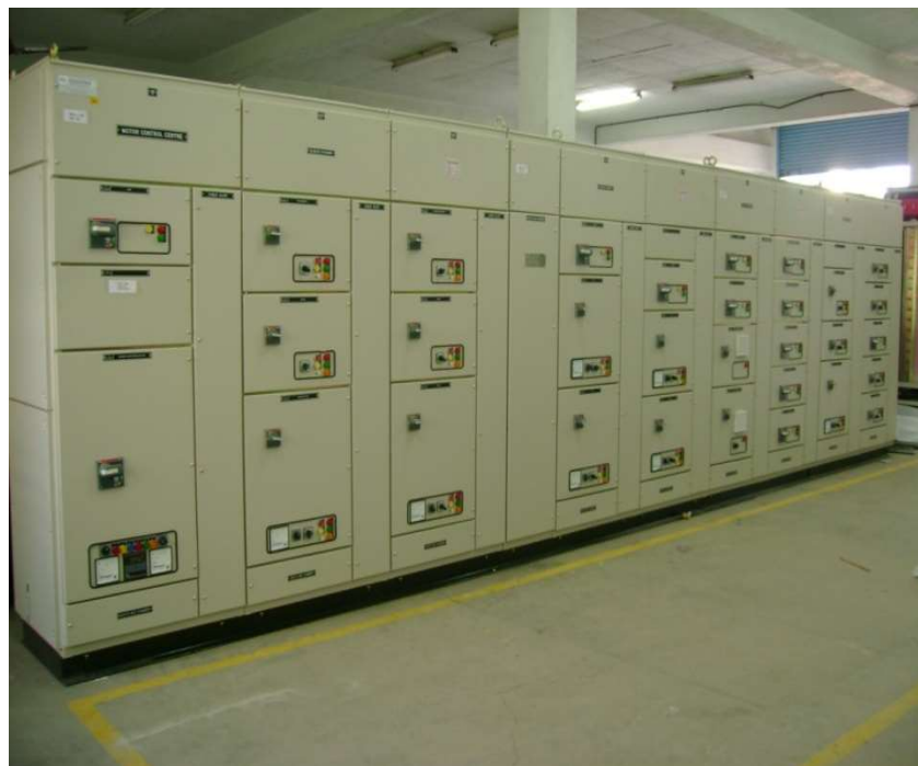
Draw-Out MCC Panel
