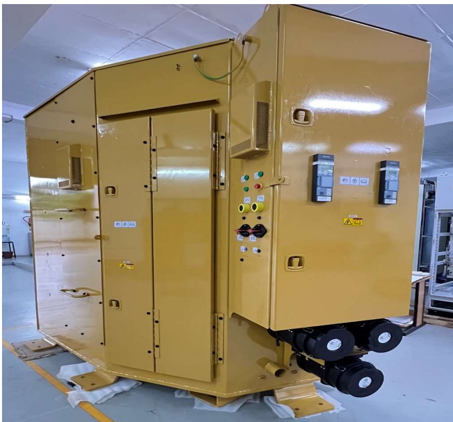
Medium Voltage Cabinet
