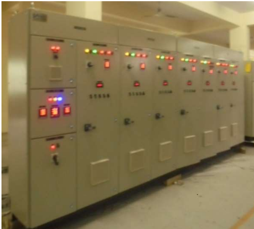
VFD Drive Panel
