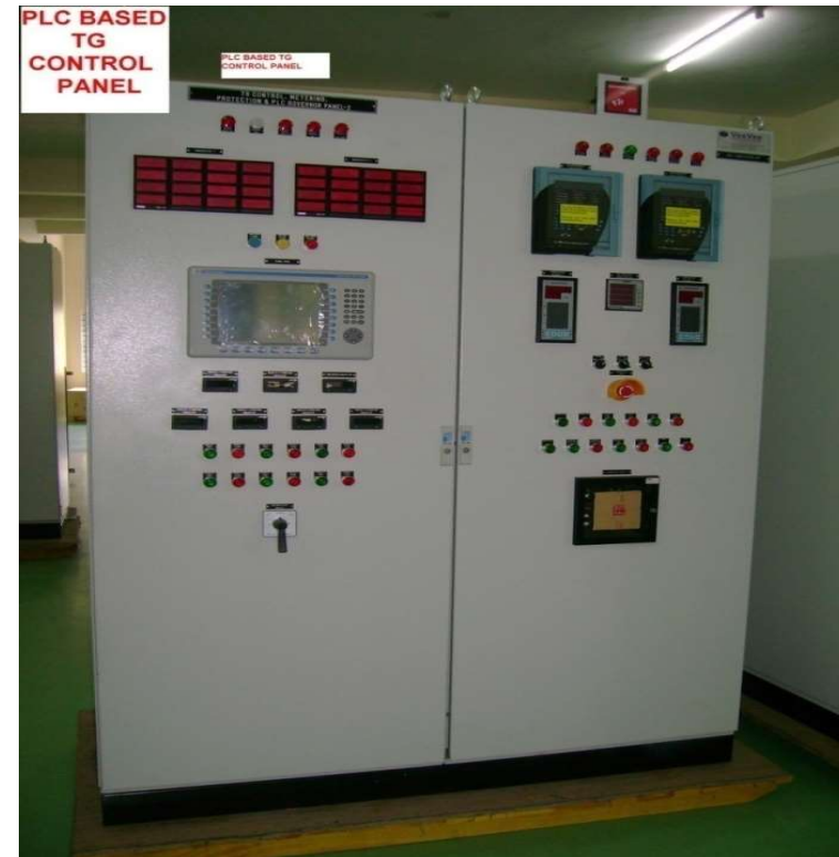
PLC Based Generator Control Panel
